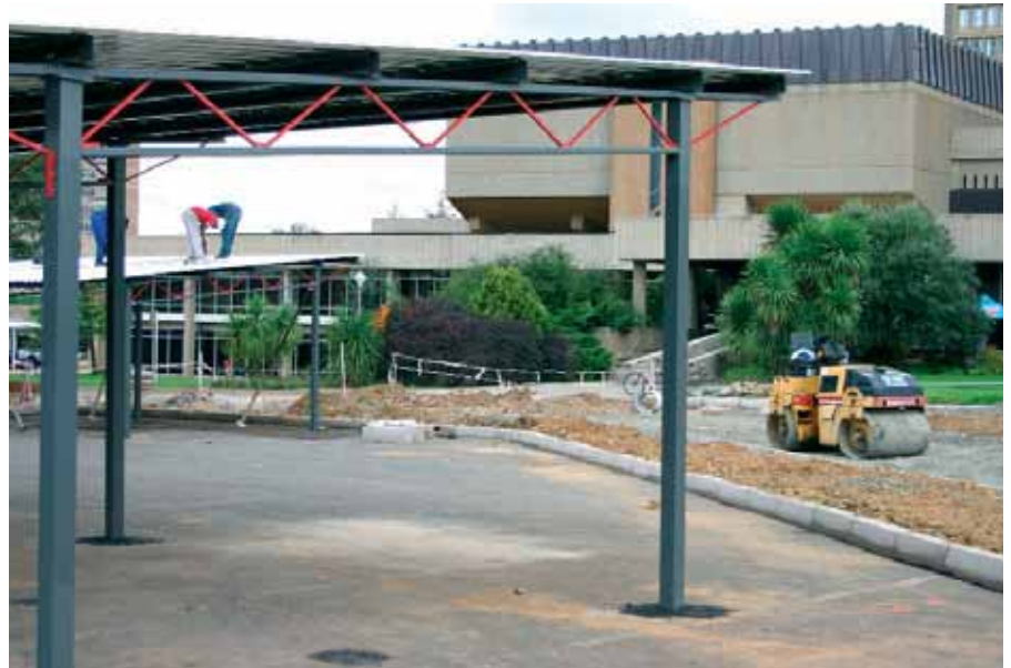
Under cover parking bays at the Faculty of Health Sciences is part of the plans for the traffic network on campus.
